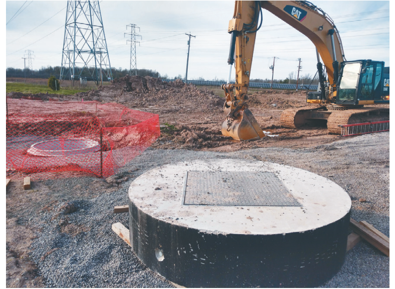
A 30-inch gravity sewer on the north side of Whitehaven Road.
